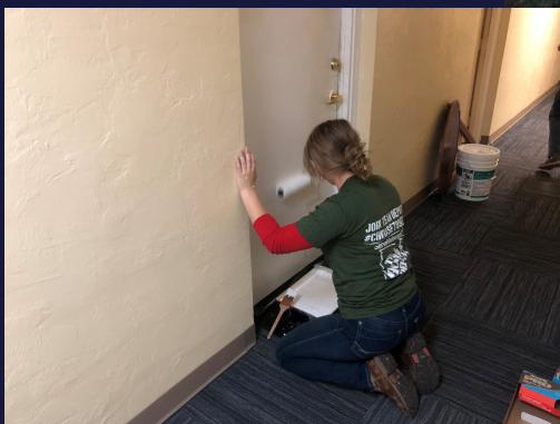
Members from The Home Depot Foundation painted hallways in our Moreau Apartments
